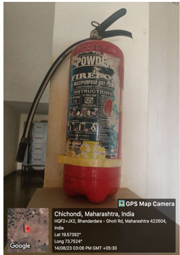
Fire Safety Equipment
