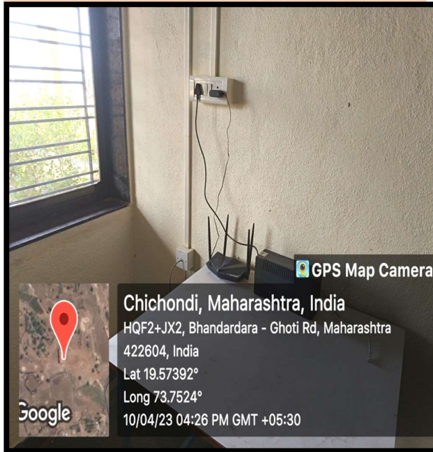
Wi-Fi Router I
